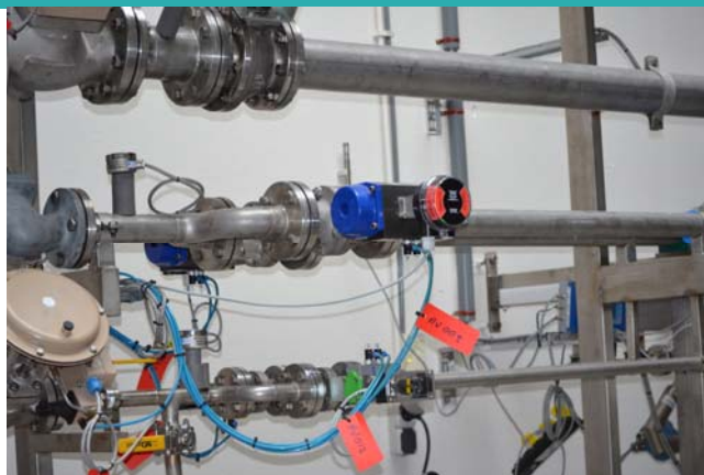
A Calibration Test Stand at VSL in Delft, the Netherlands
